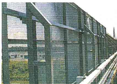
Over-Head Bridge Safety Fencing
